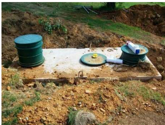
Homeowners should make a map showing the location of the components on their on-lot septic system. Photo: G. Hurd, Penn State Extension
